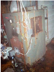
Vintage 1969 boiler, in pool of rusty water, 67% efficiency
