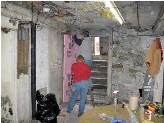
#2 — Wood hollow-core door with 1.5” rigid insulation added. “Great Stuff” foam insulation used to seal around frame and cracks in shed over stairs down. Basement ceiling had blown insulation some years back. The objective with insulation and caulking is to “fill every hole” so that cold stays outside in winter.
