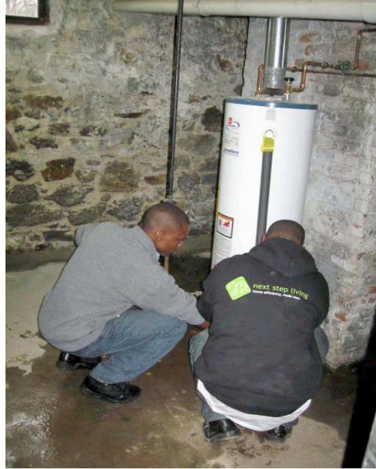
#3 — Gas-fired domestic hot water (“DHW”) tank having temperature setting lowered from HIGH to LOW. DHW was tested at the kitchen sink, and measured over 150°, which is scalding. Should be at 120°, or even less if being used for children such as at a Day Care Center. The temperature setting is an easily-understood dial, and can be adjusted by just about anybody. Setting lower – and installing low-flow aerators on faucets and low-flow showerheads — means less water and less DHW, so use reduce then cost$ reduced. Adding an insulation blanket to the DHW tank can also help, even for newer DHW tanks which are better insulated than old.
