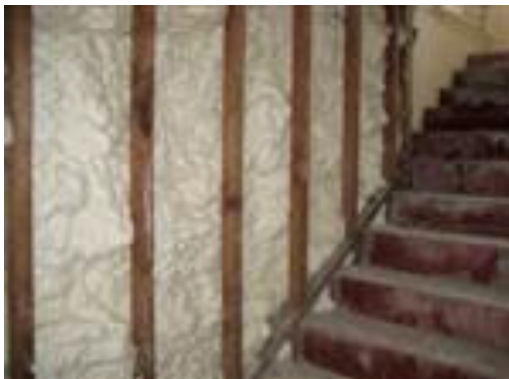
4" Icynene foam insulation was used in basement walls. All other parts of the church are insulated with either 6" or 12" blown fiberglass or cellulose fiber. Insulation ensures minimal thermal exchange between the building air and the outdoors.
