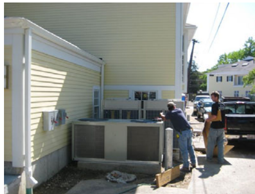
The high-efficiency HVAC (Heating, Ventilating, and Air Conditioning) system is connected to an Energy Management System (EMS) that allows the user to modify the heating schedule remotely via the Internet.
