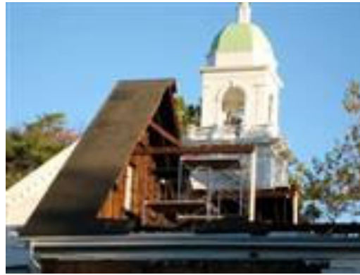
The roof over the old Parish Hall no longer met building code requirements for structural loads from snow. The new roof has a lower pitch, giving the historic Sanctuary more prominence. Roof has 12" blown fiberglass insulation.
