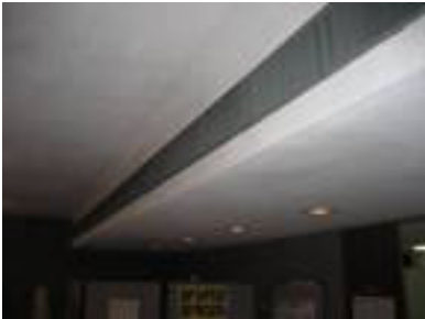
Air Ducts in the Sanctuary
