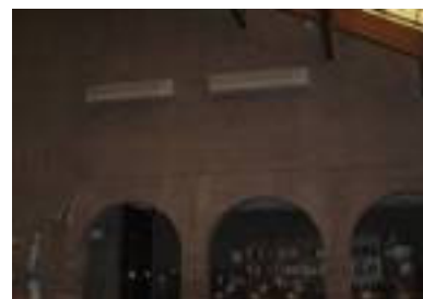
Air Handlers in Sanctuary
