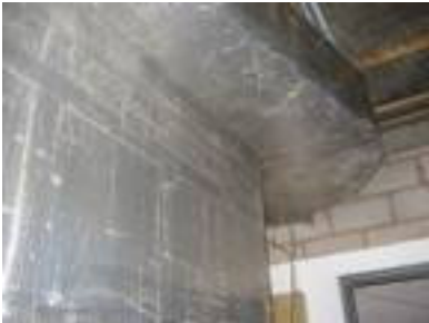
Air Ducts in Basement
