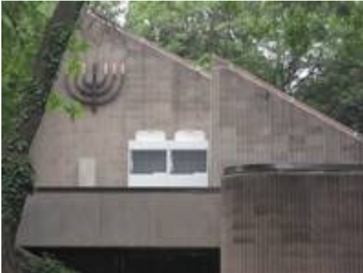
A view from the front of Boston Synagogue with the new Heat Pump
