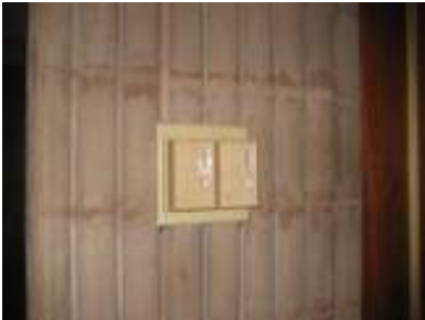
Manual Thermostats of old system
