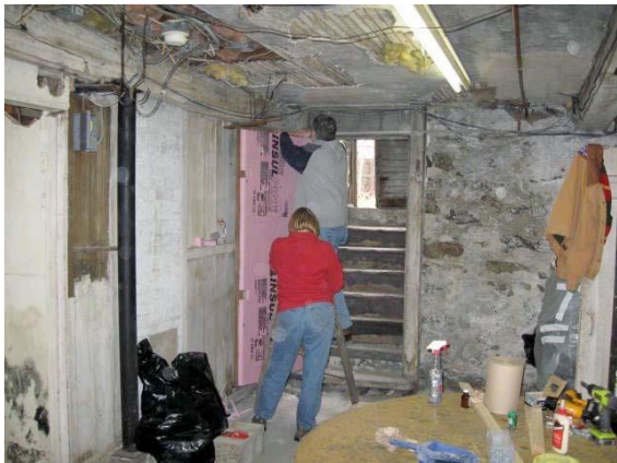
#2 — Wood hollow-core door with 1.5” rigid insulation added. “Great Stuff” foam insulation used to seal around frame and cracks in shed over stairs down. Basement ceiling had blown insulation some years back. The objective with
