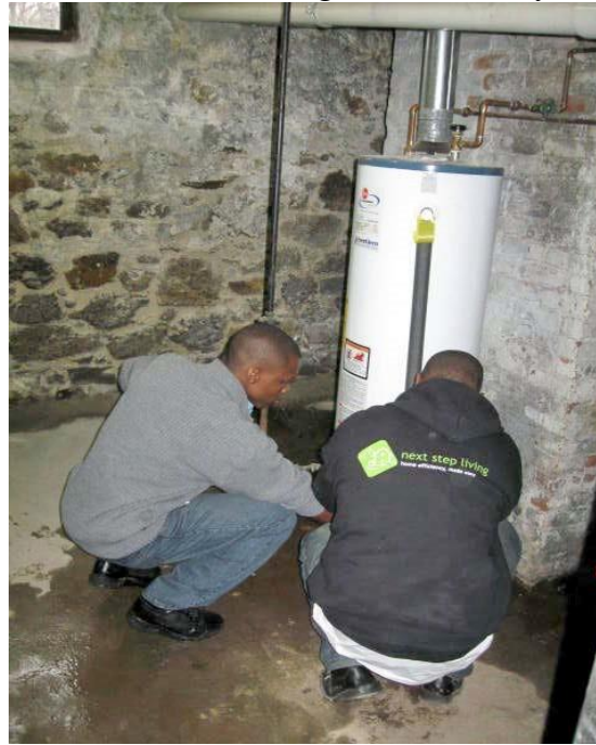
#3 — Gas-fired domestic hot water (“DHW”) tank having temperature setting lowered from HIGH to LOW. DHW was tested at the kitchen sink, and measured over 150°, which is scalding. Should be at 120°, or even less if being used for children such as at a Day Care Center. The temperature setting is an easily-understood dial, and can be adjusted by just about anybody. Setting lower – and installing low-flow aerators on faucets and low-flow showerheads — means less water and less DHW, so use reduce then cost$ reduced. Adding an insulation blanket to the DHW tank can also
