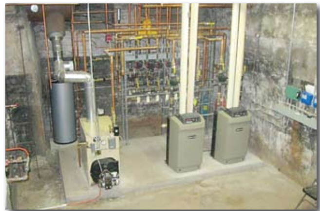
New Boilers at St. James Church.
