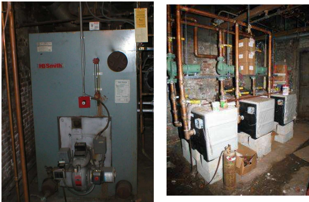
Left: Old, “dead” boiler at the Church of St. John the Evangelist, Boston. Right: Their new, highly efficient “Munchkin” boilers.
